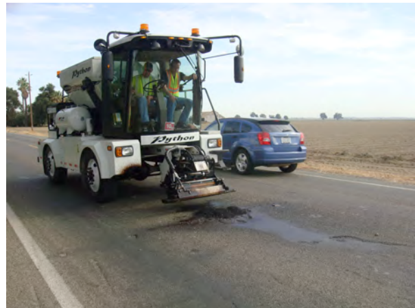
Figure 2 – Python Patching Pothole CA HWY 113
