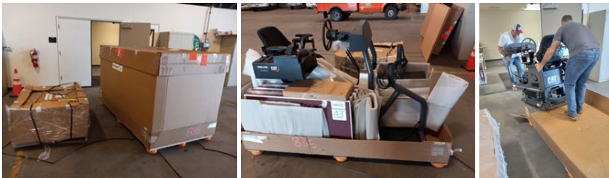
Figure 4.3: Installation of Caterpillar simulator (left and middle: transport boxes; right: sliding of based unit)
