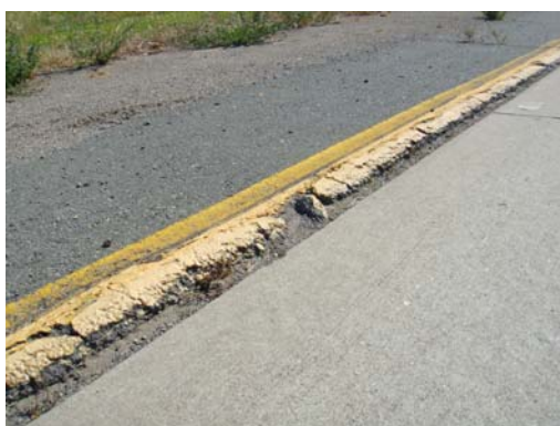
Figure 10. Shoulder Crack Lipping – Hwy 160
