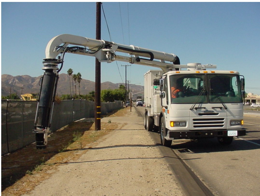
Figure 5.1 - ARDVAC positioned to collect litter on fence line
