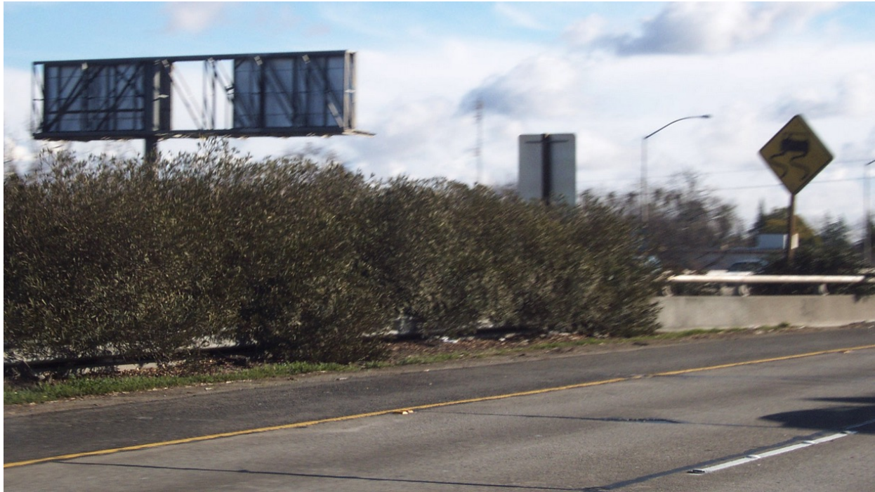
Figure 5.2 - Trash accumulating under guardrail
