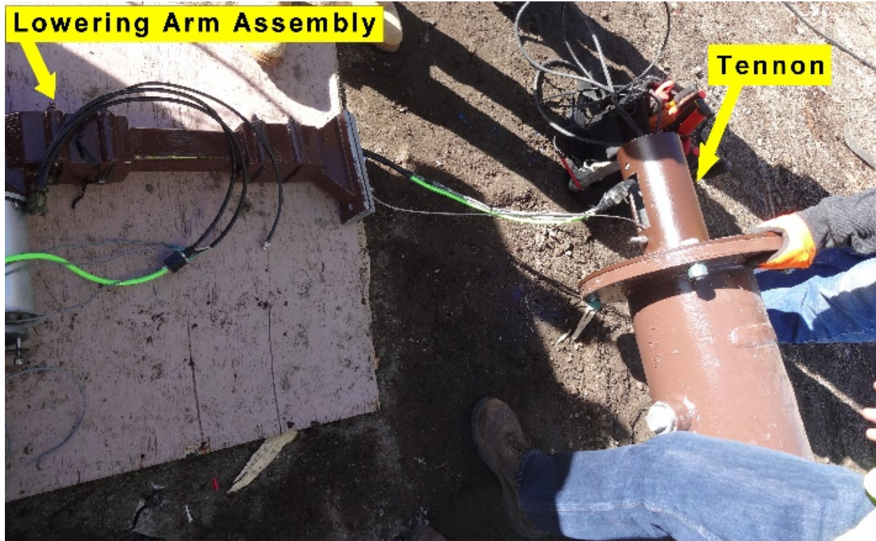
Figure 31. Pole Tenon Electrical Connections
