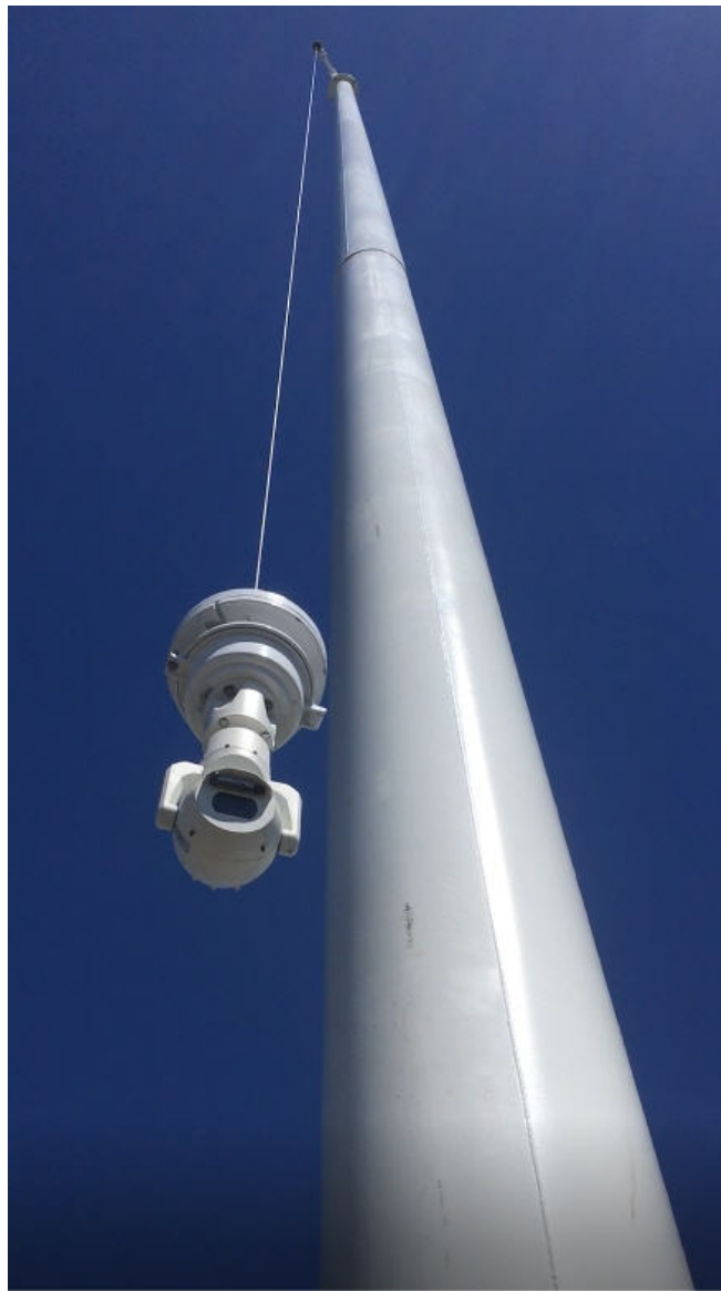
Figure 64. Bay Bridge MG 2 Internal-Type CLD
