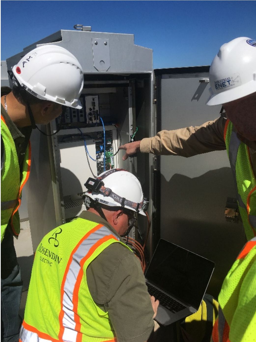
Figure 60. Bay Bridge MG2 CLD Remote Electronics Cabinet
