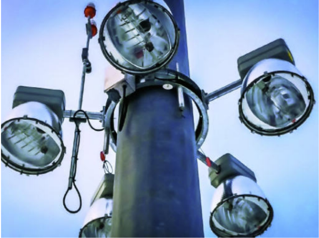
Figure 21. Halo High-Mast Lighting Application
