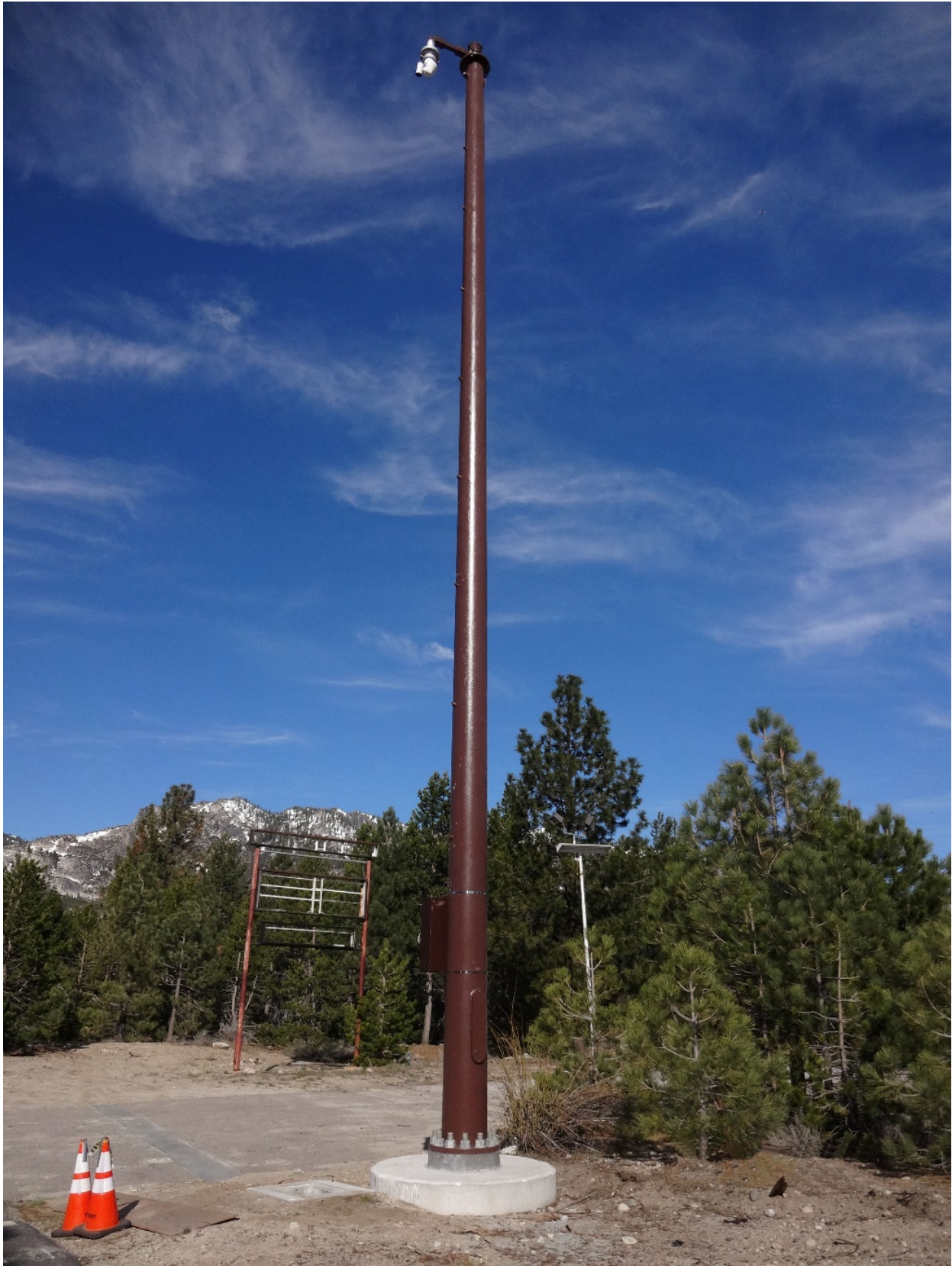
Figure 48. As-Built Meyers MG 2 Internal-type CLD Site
