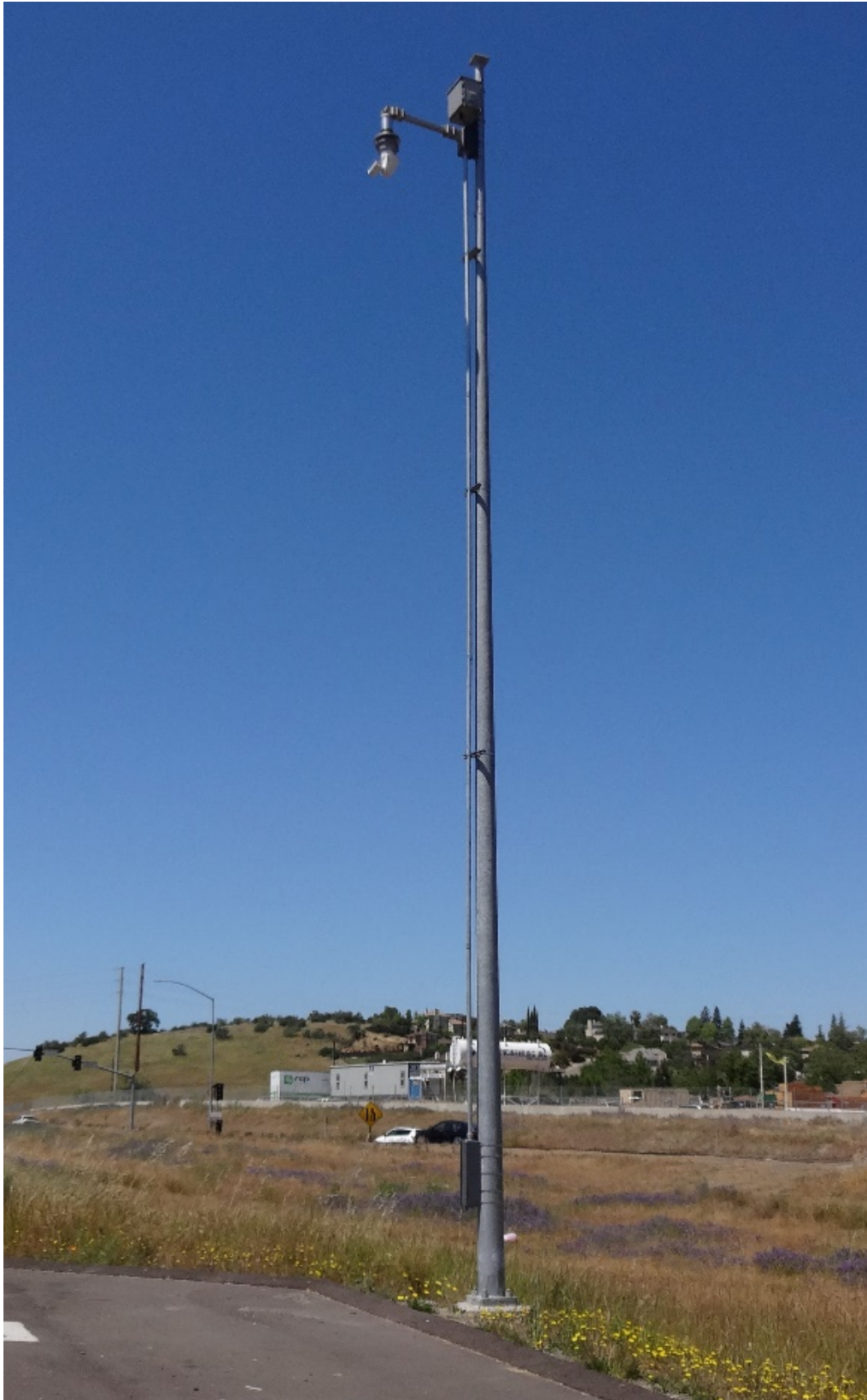
Figure 19. MG 2 External-Type CLD System, CA50 at El Dorado Hills Blvd.
